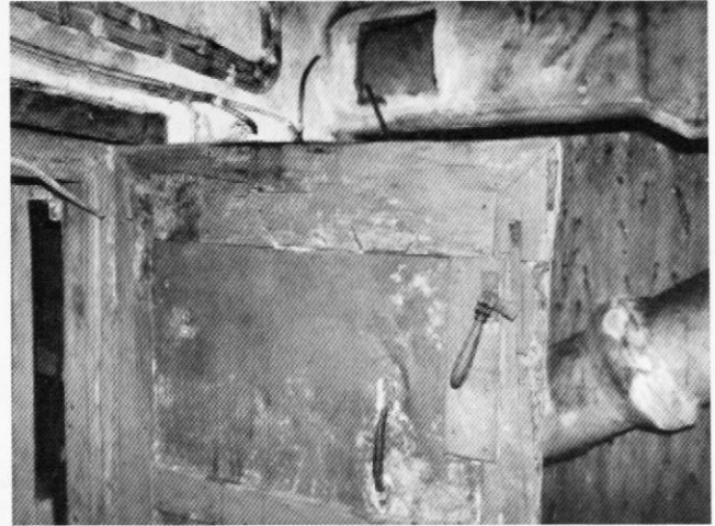
Heathfield Zero Station internal door showing closing handle and locking latch. A rubber gasket surround prevented generator fumes entering the main chamber. Air handling pipes can be seen in the background.
